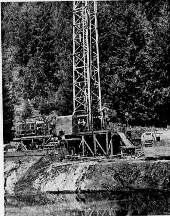
TIN-HATTED DRILLERS work around the base of the drill on the derrick. In the foreground is the slush pond where the dirt, gravel, and sand, all called "mud" by the crew, are deposited after being pumped up through the drill casing as the bit chews its way down.
