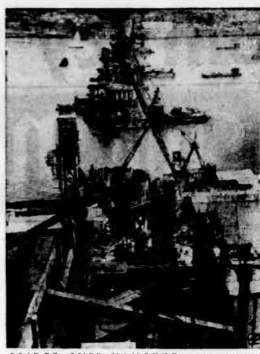
BRIDGE OVER YANGTZE — Work proceeds on first bridge spanning the Yangtze River at Wuhan in south central China. Construction is supervised by 20 top Soviet engineers.
