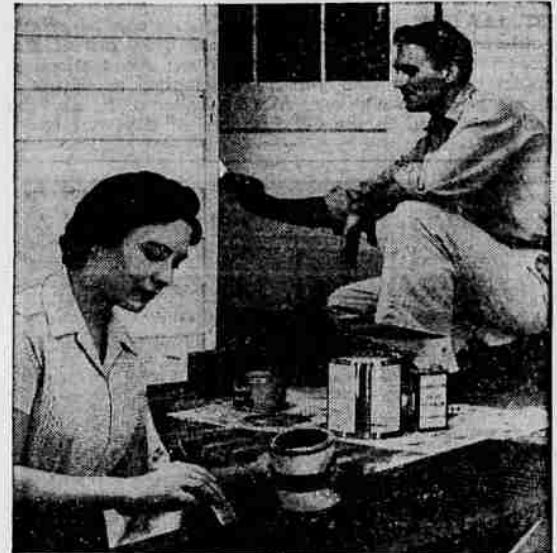
BEFORE THE FINISH COAT is applied, all surfaces must be carefully prepared. Rough spots should be sanded smooth, all rust removed. Cracks should be filed. Any spots of bare wood or metal must be primed.
