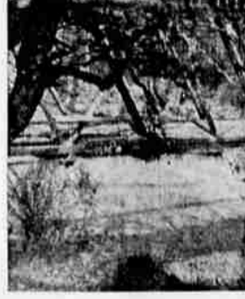
END OF LINE—County bridge crews are dismantling the old Rice Bridge east of Dillard because three floods and an arson attempt had made the span unsafe. Though it doesn't appear so here, the structure was one of the few remaining covered bridges in Douglas County. The County Court hasn't decided whether to rebuild. Engineers estimate replacement would cost about $100,000. (Paul Jenkins photo).
