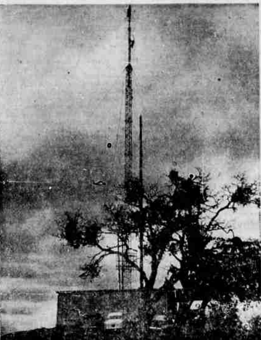
ANTENNA IS UP — Workmen finished the last major piece of work on the KPIC-TV antenna Friday and then sent the more than 150-foot structure skyward. Antenna will beam television to Douglas County sometime before Feb. 15, it is anticipated. The tower and its tall lanky addition are located on Rose Mountain, northeast of Roseburg. The site is 1,700 feet above sea level. (Paul Jenkins picture).
