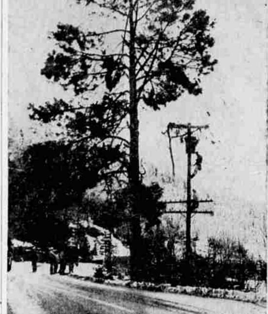
DISRUPTED power service in the Glendale area has been restored, however some telephones are still out of order in the region south of Glendale. Earlier in the week a large limb fell on power lines east of Glendale. Witnesses said that smoke from the hot wires billowed in black columns until Copco workers could be informed and cut off the power. Pictured above, an unidentified Copco worker cuts the limb to clear the lines, while Bob Jones, manager of the Glendale telephone exchange, waits beside the cross arm below to help prevent damage there. (Fox photo).
