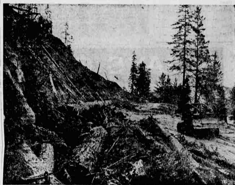
LOGS AND OTHER DEBRIS litter the roadbed on Highway 38 near where a bulldozer and donkey operate a bucket to pull mud and rocks from overhanging bluff.
