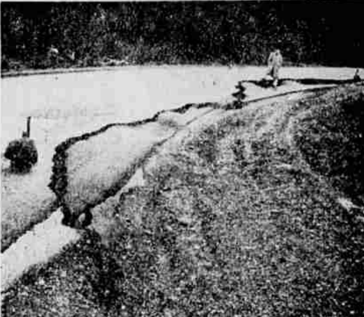
ROAD DAMAGED—Water soaked the bed of the Lookingglass Road near the summit between Roseburg and Lookingglass, and this section of pavement slipped away from the rest of the grade.
