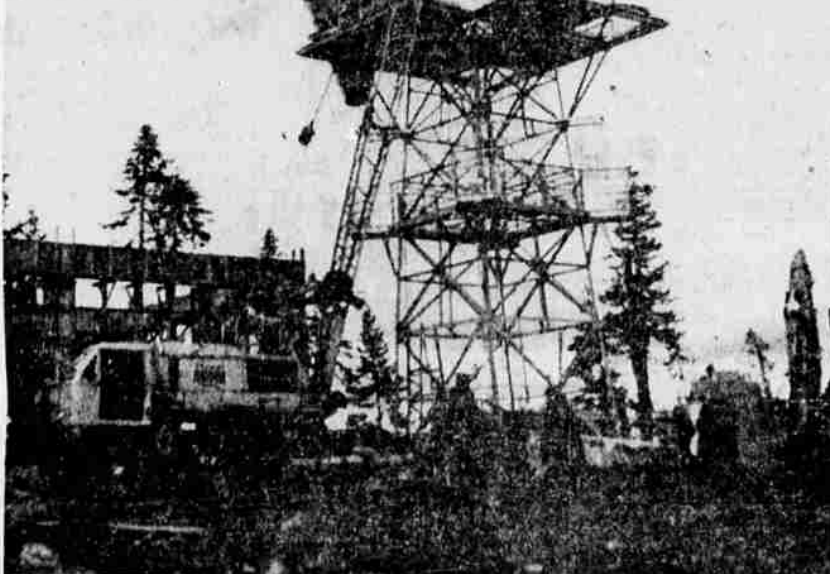
HIGH IN THE SKY — Microwave antennae to provide channels for transmission of network television programs are being installed atop King Mountain, some 80 miles southeast of Roseburg. Delicate apparatus stands 22-foot tall and is placed on 37-foot tower on the 4,800-foot mountain.
