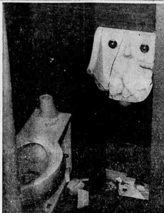
JAIL CELL DAMAGED — Two youths charged with armed robbery used table legs to smash plumbing and windows in their cell in the county jail Monday evening. This is a typical example of the damage done. The rioters were Robert Eugene Mitchell, 18, and Richard Allen McKelvey, 17, indicted by the grand jury in the gunpoint robbery of a Myrtle Creek grocer Aug. 30. (Mindolovich photo).
