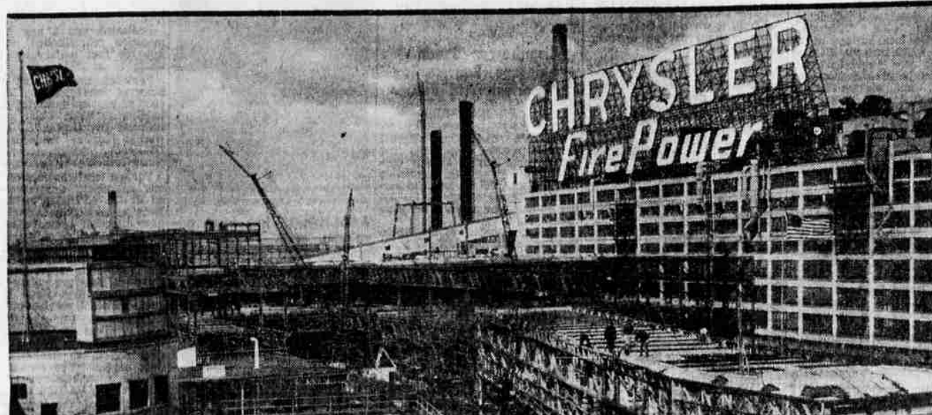
UP GOES CHRYSLER'S PRODUCTION MORE THAN 40% Here you see construction work proceeding on the new Chrysler production facilities which will add 667,000 square feet of floor space... including a 1 1/4-mile long continuous conveyor system, longest in the industry.
