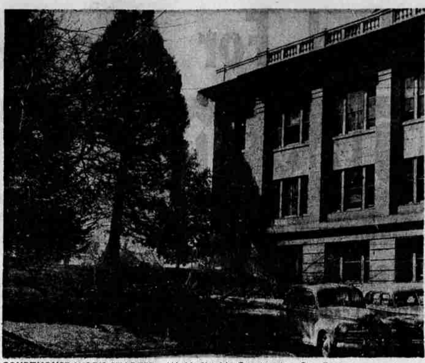
COURTHOUSE WORK STARTED—W. H. Shields Construction Co., Eugene, general contractor in the building of two new wings to the Douglas County courthouse, started work this week by felling trees on the grounds. Work on the east wing, above, will be started first. Excavation is next. (Paul Jenkins photo)
