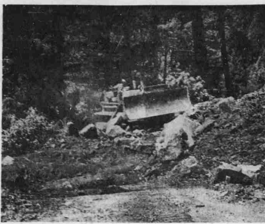
DELAY AHEAD —Motorists on the North Umpqua Highway between Steamboat and Apple Creek may be confronted with a scene like this during the next few months. The road, where construction is being handled by the Bureau of Public Roads for the Forest Service, will be closed periodically each day through the remainder of the summer. The terrain offers no opportunity for a detour route, so travelers may have to wait at certain times when blasting or grading are under way. The roadwork will be a boon to the Umpqua Valley, however, because of better access to timber. (Picture by Paul Jenkins).
