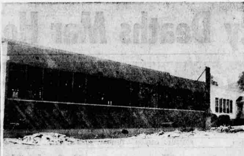
GOING UP—The new Days Creek High School is shown above at its present stage of building. The $72,000 structure will probably be completed by Aug. 1. (Story Page 12).
