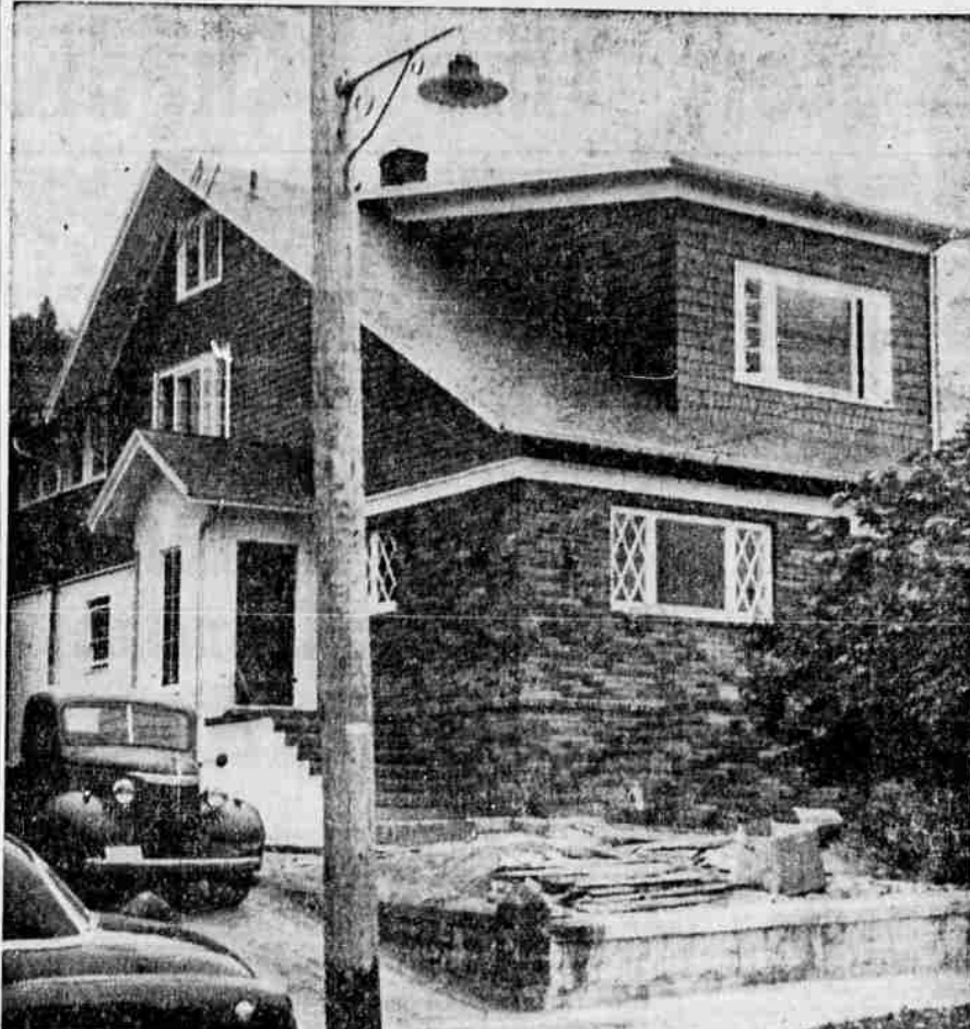
HOME REMODELED — The former Clay Darby home, above, on Kane Street between Washington and Douglas, is being remodeled into a residence and three apartments by its purchaser, William Harris. The house was first built about 1912, and is now being renovated both inside and out. (Picture by Paul Jenkins)
