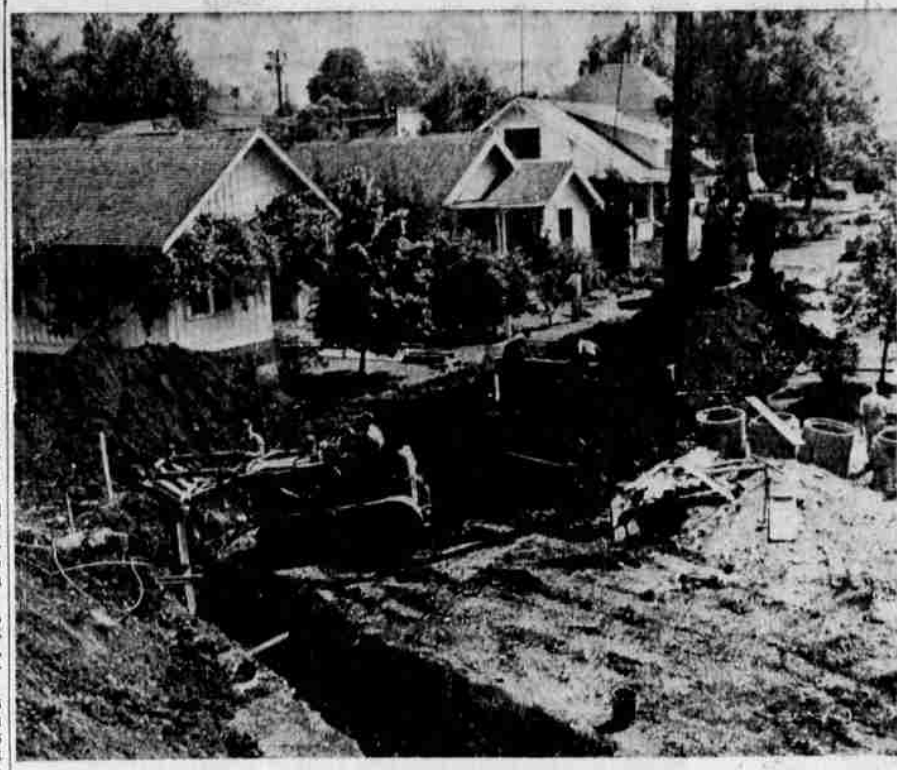
NORTH JACKSON storm sewer project, under contract to Stoneburner Construction Co. of Springfield, was started this week on Rowe St., near the N. Stephens St. bridge across Deer Creek. At this point the storm waters from the north part of town will drain into the stream. (Paul Jenkins picture).
