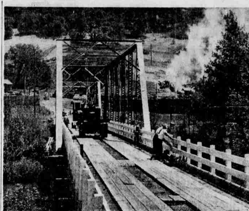
MARY MOORE BRIDGE on the Round Prairie road crossing the South Umpqua River is shown above as workmen began taking off old plank decking this week to replace with steel plates. The bridge, built in 1925, will be slightly wider with the new steel deck. County officials said the span would be closed to traffic for three to four weeks during the construction. West Coast Steel Works is doing the work under contract from Douglas County. (Picture by Paul Jensen).
