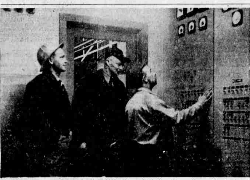
FORESTER INSPECTS POWER DEVELOPMENT — J. Herbert Stone, forester for the North Pacific region, embracing Oregon and Washington, is pictured, center above, as F. L. Mercate, powerhouse operator, explains operation of the remote control panels governing the Slide Creek generator from Toketee powerhouse. Phil Humphreys, left, is superintendent of Copco's hydroelectric project in the North Umpqua district. Forester Stone made a brief inspection of the Umpqua National Forest as far as Toketee Thursday.
