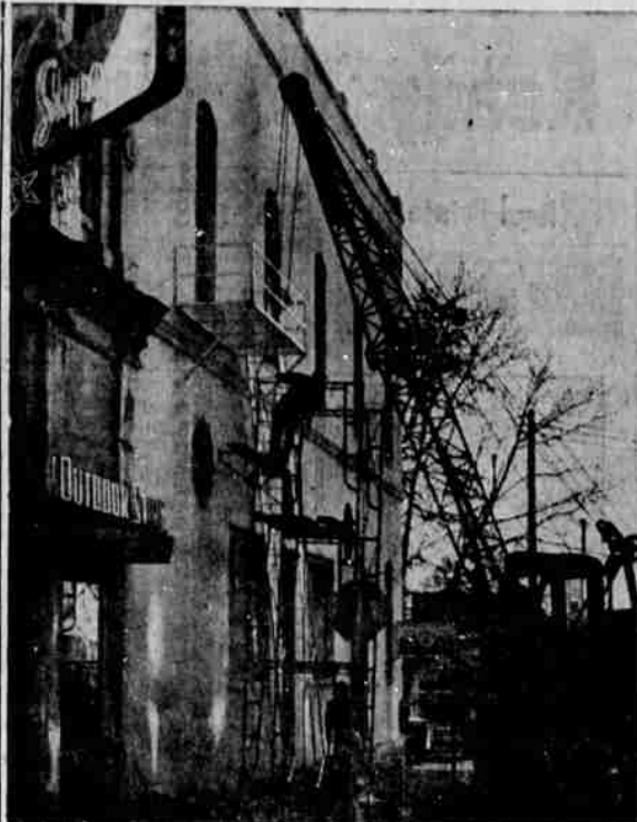
THE MASSIVE CRANE holds the steel fire escape, above, while welders affix it to the side of the Hochradel Building at the corner of Jackson and Washington Streets.
