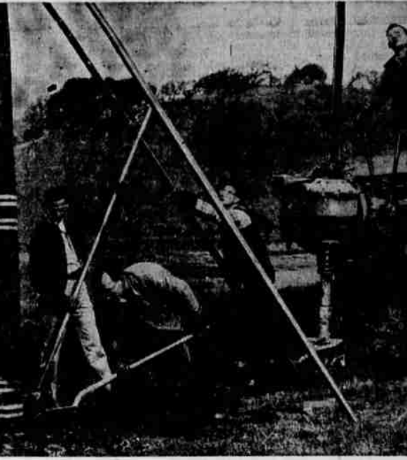
"Pole stubbers" at work: Inspection has revealed a pole which shows damage at the ground line. Now, reinforced with a short length, it will be strong as new, and we'll have saved much of the cost of a new pole.
