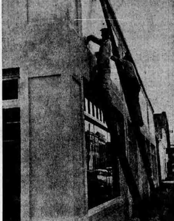
JOSEPH H. De ROSS, on the ladder at the left above, and his companion, Clyde Bluejacket, are shown busily engaged in painting the exterior of the Oregon Supply company at Main and Washington streets. Carl Cornell, their employer, has the contract for the job. The color, a light turquoise, was chosen by Bill Oeding, owner of the Supply company, over Carl's violent protest — "color is more fit for a parlor than the outside of a business building, etc." but so many compliments have been received concerning it that Bill believes even Carl is weakening a bit and pretty soon may come actually to admire it — he hopes.
