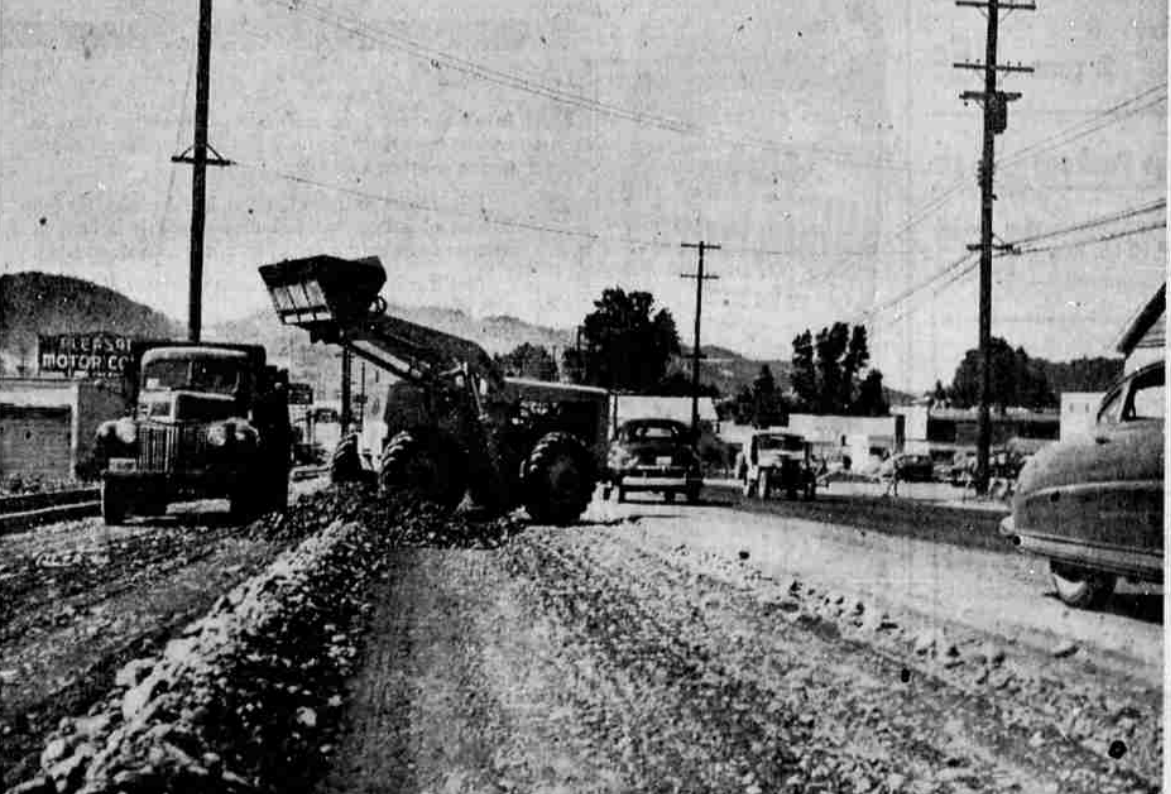
HIGHWAY 99 IMPROVEMENTS—Paving work is progressing on the four-lane highway from the north Roseburg city limits to the Garden Valley road junction. The right panel of the highway, looking north in the picture is already paved. The center strip is ready for paving, and the left strip is now being prepared for black top surfacing. (Picture by Paul Jenkins)
