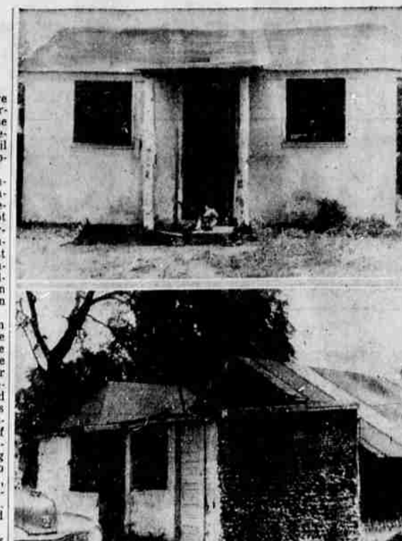
These are two of a number of pictures of substandard housing for service men and their families published in an interim report on substandard housing and rent gouging of military personnel by the preparedness subcommittee of the senate committee on armed services. At top is "The Box," a tiny shack in the Camp Breckinridge, Ky., area. Divided into two small rooms, it rents for $20 a month to a sergeant, his wife and child. At bottom is the "Bottle House" constructed of whiskey bottles, beer cans, oil cans and mortar. A corporal and his family of three pay $25 a month rent. (AP wirephoto).
