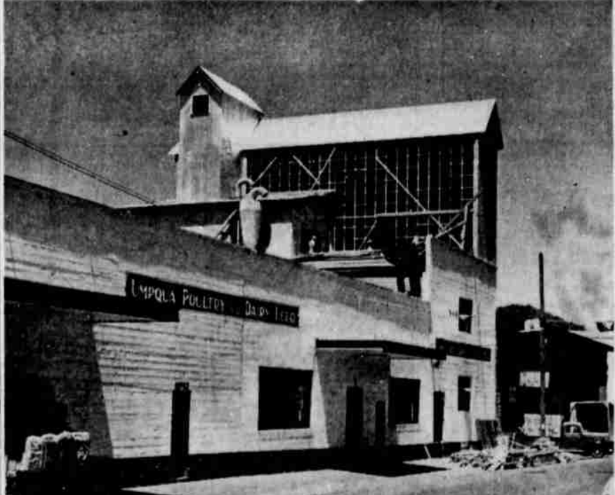
MORE SPACE—Pictured above is the addition (at right) now under construction at the Douglas County Flour Mills by the Todd Building company, increasing elevator and storage capacity for grain at the mill by 50 percent, or to 16 fifty-ton carloads. (Picture by Paul Jenkins)
