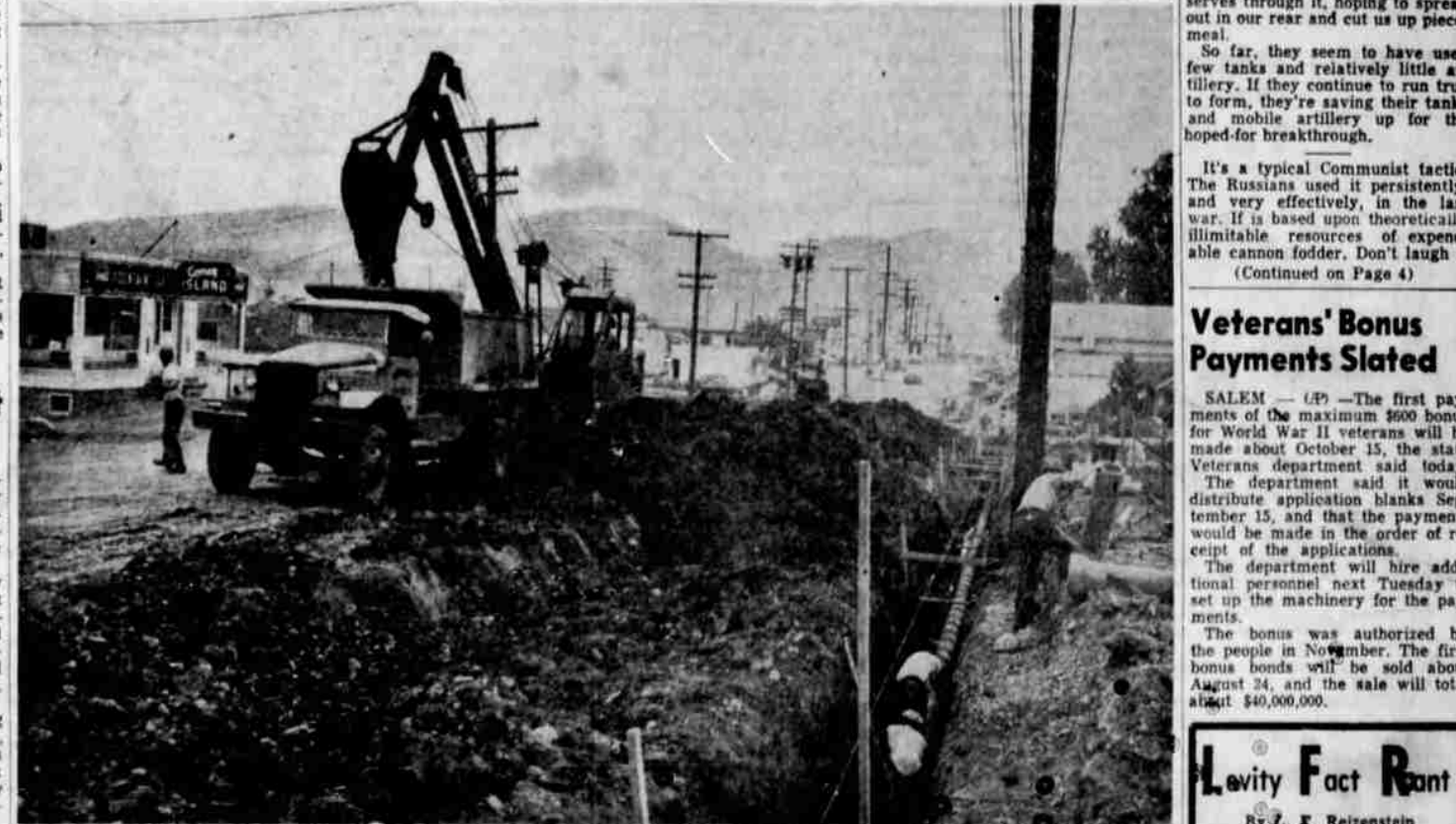
CONSTRUCTION PROGRESSES — Things are really humming along the highway in North Roseburg these days. Pictured above is a Pre-Mix concrete truck taking on a load of earth, while workmen are laying pipe line for the North Roseburg sewer project. The state highway department, under a contract let to K. F. Jacobsen Construction Co., is doing preliminary work toward the construction of a four-lane highway from the Roseburg city limits to the Garden Valley Road junction. Drainage tile is to be laid beneath the highway, and the telephone company is also laying underground cables in the area. (Picture by Paul Jenkins.)
