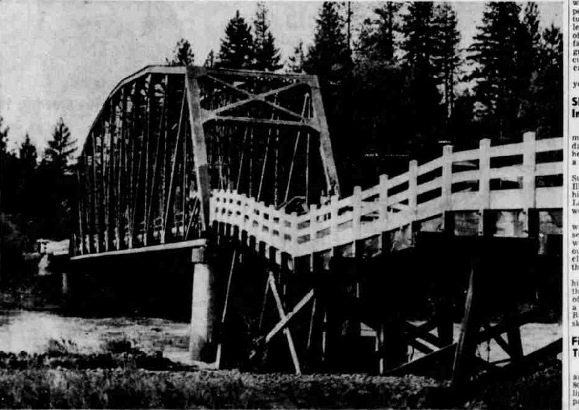
THE SOUTH APPROACH to the bridge near Ford's at Canyonville on the South Umpqua river was seriously damaged by the flood Sunday. The underpinnings of the approach were ruined by debris carried by the flood waters. The bridge was restored to temporary use today. (Picture by Paul Jenkins.)
