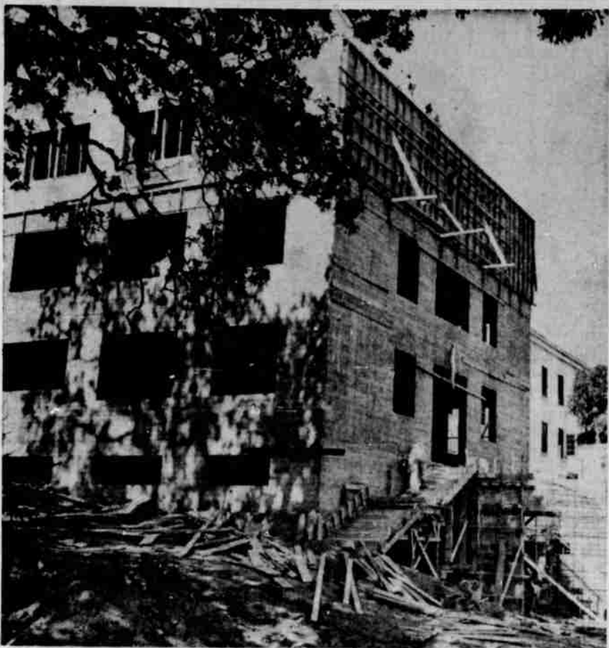
CONSTRUCTION PROGRESS —The west, or service, entrance to the new Mercy hospital unit, now under construction is shown above. Construction of the unit has been going ahead with available funds, awaiting final approval of a federal grant. Assurance that the money will be forthcoming has been received by the hospital management. (Picture by Paul Jenkins.)
