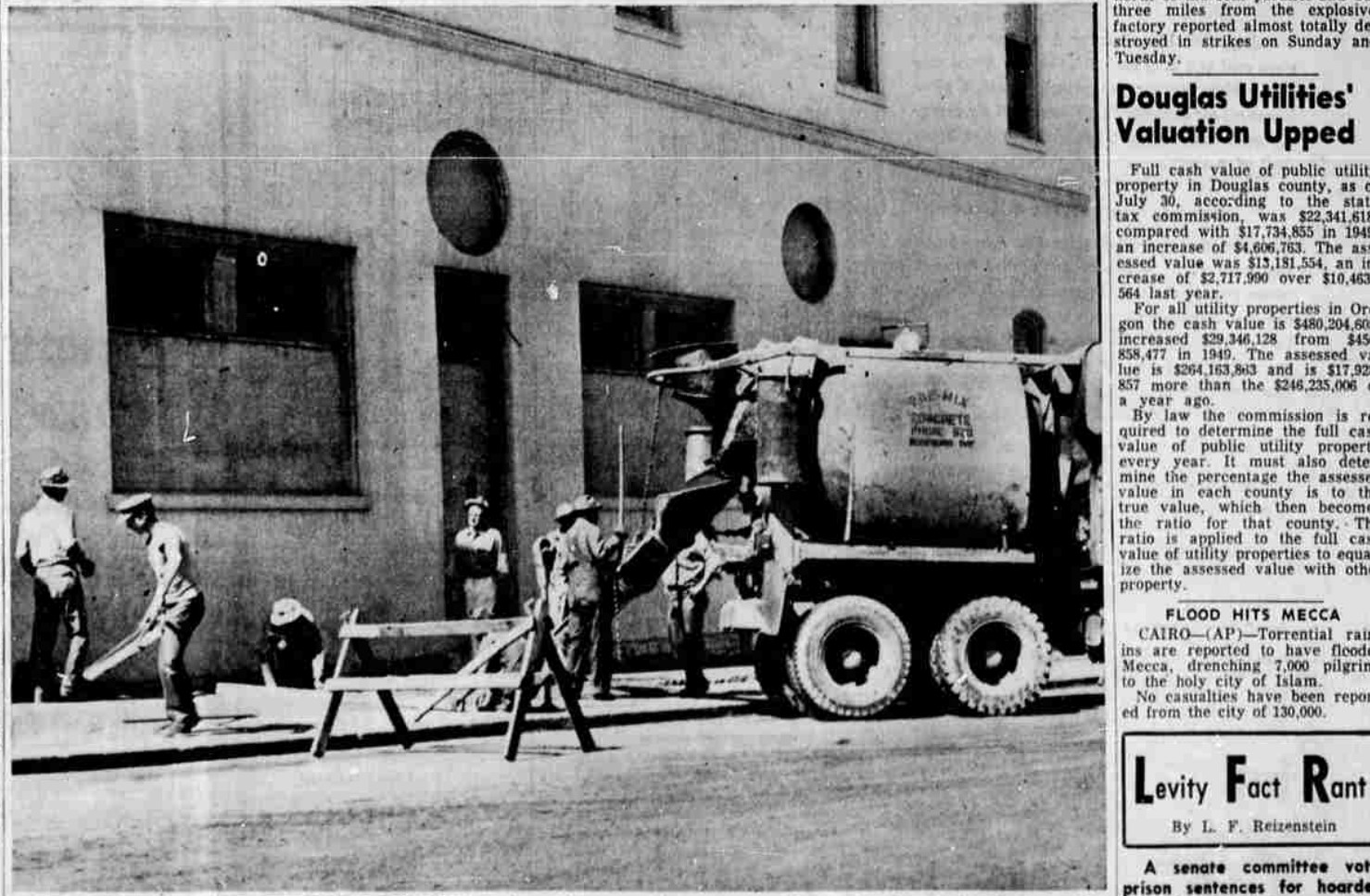
PACIFIC TELEPHONE AND TELEGRAPH COMPANY workmen are shown repairing portions of the sidewalks and street, torn up for the installation of underground exchange service cables. R. J. Henwood, local manager, said this is part of the company's program to put under ground all possible telephone lines, to eliminate unsightly overhead wires in the main business section. Lines have been extended down Mosher, Washington and Rose streets and other important sections. (Picture by Paul Jenkins.)
