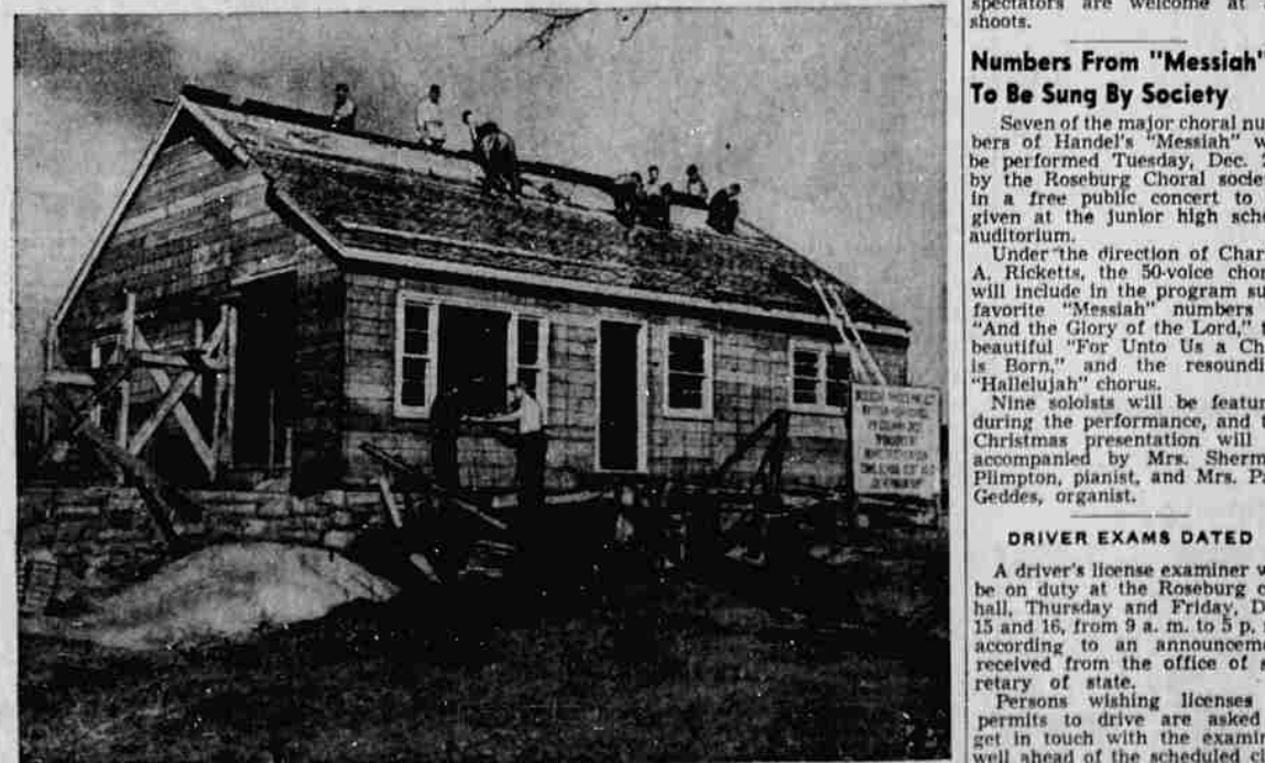
STUDENT PROJECT —Students in the building trades class of Raytown, Mo., High School, work on the six-room house with garage they are building as part of their class work.
