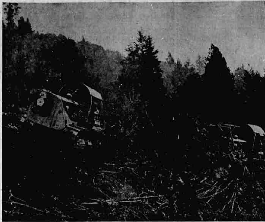
GIANT TRACTORS team up in the clearing of right-of-way for the re-construction of the Pacific Highway through the tortuous and rugged canyon between Canyonville and Azalea. Building of the section extending from Deer Park Inn, in the lower canyon, to Azalea has been awarded to the Kuckenber Construction company of Portland by the State Highway commission at a bid of $1,200,000. This firm has commenced clearing operations at the Pioneer bridge and also at a point just south of the summit.—(By Paul Jenkins).
