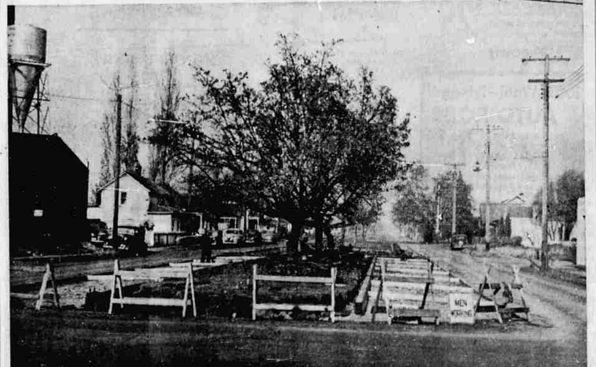
NO. JACKSON ST. WIDENING—Illustrated here is the start of a program which will eventually result in the widening of No. Jackson street's traffic lanes its entire length. However, limited funds make possible that the work be done piecemeal. Under construction now is the widening of the one block north of East Second Avenue So. From this street to the railroad tracks, the parking strip is being cut away 12 feet on either side. This will widen to 28 feet both lanes of traffic. From the railroad track north to East First Avenue south six feet is being lopped off both sides of the parking to provide a 22-foot street width on either side. The parking strip originally was 44 feet wide.—(Picture by Paul Jenkins)
