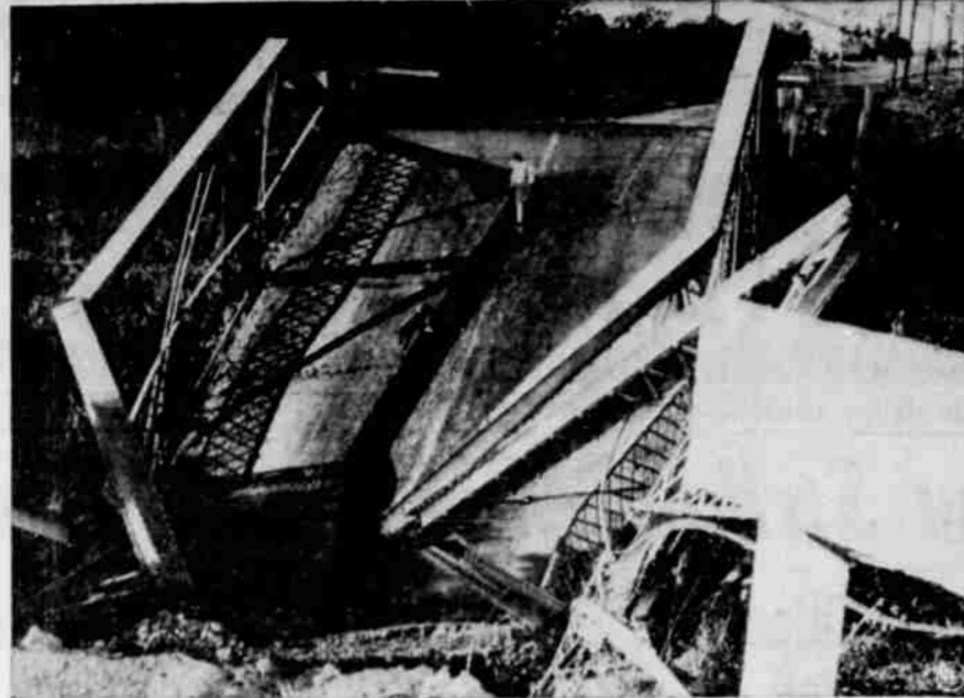
ALL OF A SUDDEN IT COLLAPSED—The wonderful one-hoss shay had nothing on this 50-year-old bridge near Stockton, Calif., except an extra fifty years. The 70-foot steel bridge just collapsed, for no apparent reason, and with no one on it at the time. Evidently it had just used up its allotted span. When the photographer found it, it was being used as a romping ground by a small boy and his dog.
