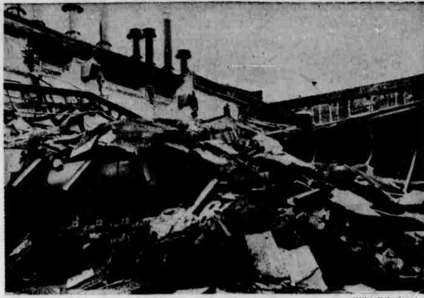
BLAST WRECKS POWER PLANT —Turbine room of a million-dollar power generating plant at Rushville, Ind., lies in ruins after a diesel engine developed a hot piston and blew up. Two men were killed in the blast. The plant provided electricity for 11 counties.
