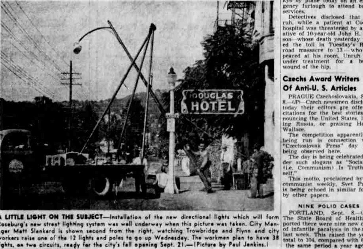
A LITTLE LIGHT ON THE SUBJECT—Installation of the new directional lights which will form Roseburg's new street lighting system was well underway when this picture was taken. City Manager Matt Slankard is shown second from the right, watching Trowbridge and Flynn and city workers raise one of the 12 lights and poles to go up Wednesday. The workers plan to have 38 lights, on two circuits, ready for the city's fall opening Sept. 21.—(Picture by Paul Jenkins.)
