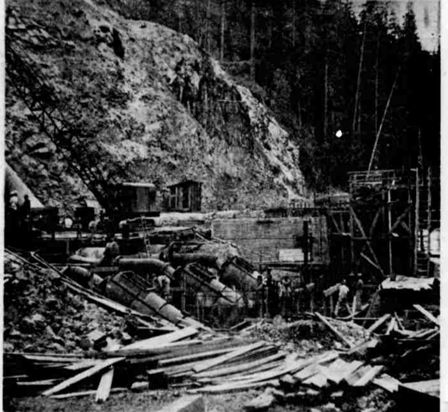
POWER PLANT PROGRESSES—The three photos above indicate the progress being made at Copco's Toketee falls project on the North Umpqua river, 65 miles east of Roseburg. Top view shows the three penstocks which will bring water to the powerhouse from the mouth of the 5,300-foot tunnel, approximately 400 feet above the powerhouse site. Center picture is a downstream view of the powerhouse site. Equipment predominating in the photo are the bypass conduits, which will permit a flow of water to be maintained around idle turbines. Force of the fall is broken before water is released into the spillway. At left center of the middle photo may be seen the circular base upon which will rest one of the three turbines. Water to the turbine will come from the flanged pipe seen at extreme right center. Lower photo presents an overall view of the powerhouse site, looking upstream, showing the level of the concrete floor to be built over the equipment now being installed and on which will rest generating equipment. (Staff pictures.)
