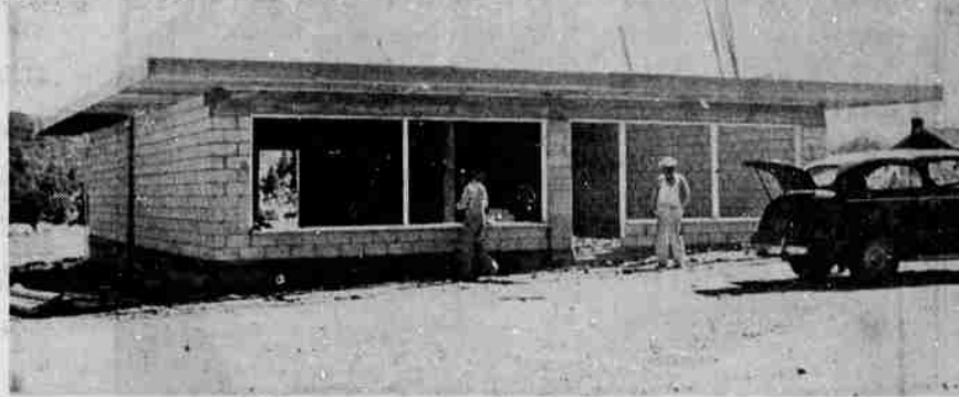
NEW BUSINESS RISES —Occupying a portion of the familiar circus and carnival grounds on Garden Valley road is this new building, which is being erected by O. B. Digby to house a drive-in food market. Digby plans to operate the business himself under the name of Digby's Food Market. The building when completed will include a 20-foot extension on the rear, and 26 by 40 foot quarters above the store. Digby erected a drive-in market bearing his name north of the city in 1937, but sold the business in 1944. (Picture by Paul Jenkins.)
