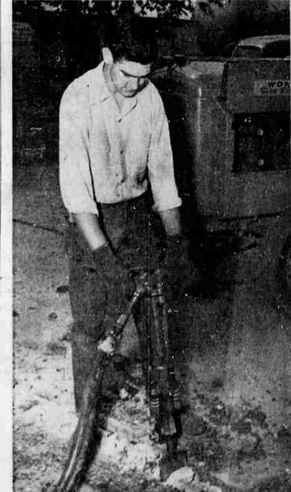
STREET LIGHTING SYSTEM —Roseburg's new street lighting system will soon become a reality. The above pictures show the preliminary work underway. Much of the work of installing such a system is underground. The general public sees only that which is overhead, but little realize the actual work of total installation. The picture on the left shows Edward Stinson with an air drill cutting the sidewalk pavement on West Oak Street for the laying of electrical conduits. The picture on the right shows connections, pipelines and conduits to the street lamps on West Cass Street. Trowbridge Electric, under the direction of Ray Simms, has contracted to do the work. Total of 115 lights will be installed. (Picture by Paul Jenkins.)
