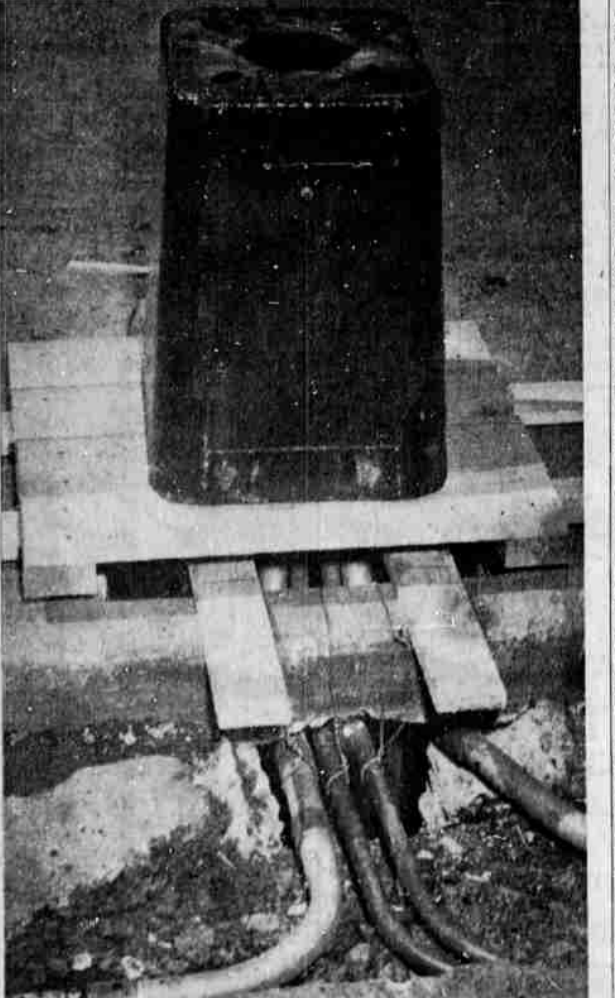
The picture on the right shows connections, pipelines and conduits to the street lamps on West Cass Street. Trowbridge Electric, under the direction of Ray Simms, has contracted to do the work. Total of 115 lights will be installed. (Picture by Paul Jenkins.)
