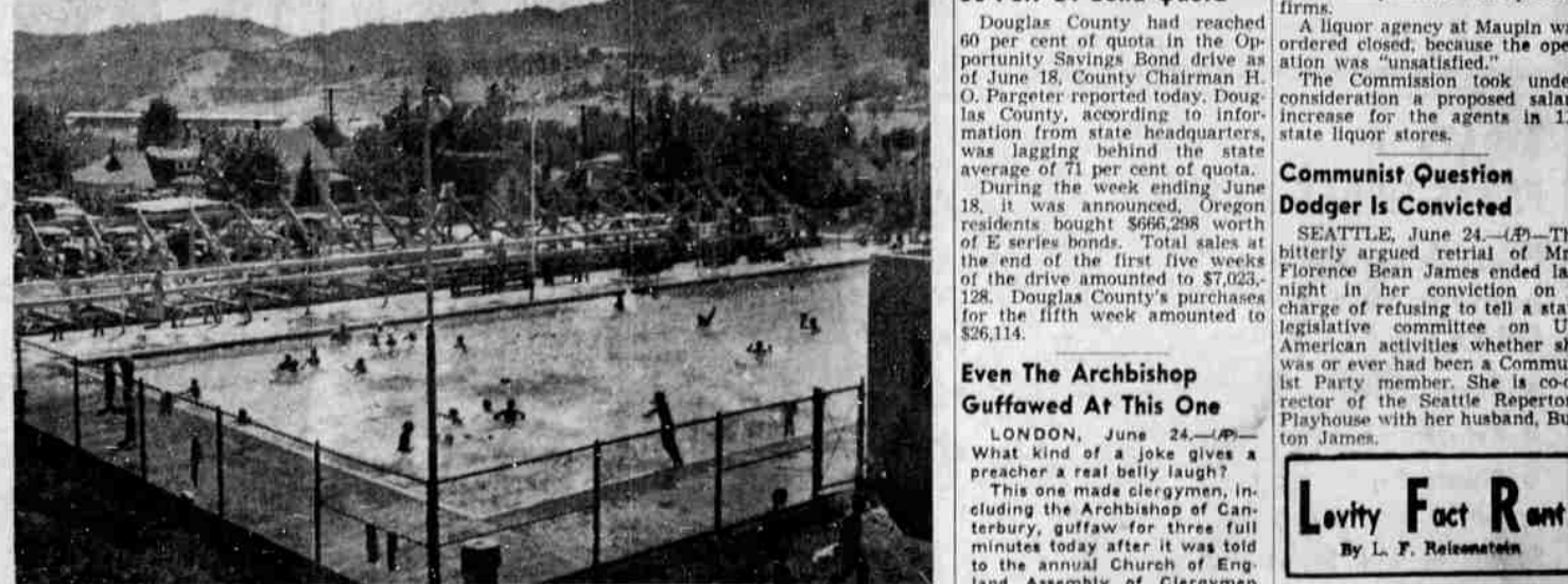
BLEACHERS INSTALLED—The final step making it possible to conduct major swimming meets in Roseburg has been taken with the erection of bleachers along the south side of the municipal pool. M. W. Sliankard, city manager, said the bleachers would be completed this week. The Junior Chamber of Commerce's plans for the big water festival here July 9 and 10 are shaping up well, and some outstanding amateur swimmers are expected here for the event. (Picture by Paul Jenkins).
