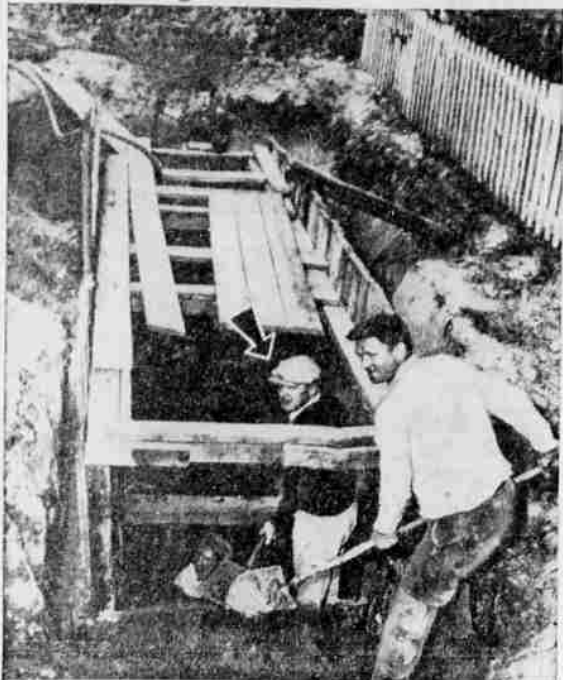
Keeping his campaign promise to provide a better sewer system, Raymond O'Brien (arrow), president of Hazelcrest Village, a suburb of Chicago, works in a ditch with other village officials. Working evenings and weekends without pay, O'Brien and his colleagues expect to save the community two-thirds of the usual cost of the job.
