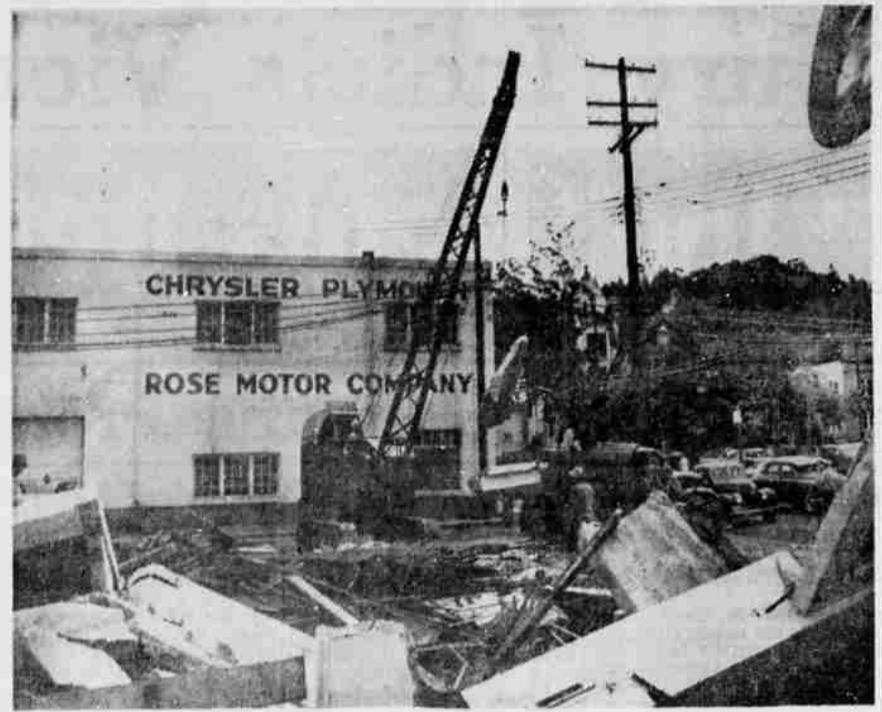
PROGRESS—This was all that remained Friday of the once proud Union Oil Service Station at South Stephens and Lane Streets. The station, built about 1920, was one of the oldest, if not the oldest, service stations in Roseburg. Constructed of reinforced concrete, it was a sturdy building, but not modern, and such buildings cannot stand in the way of progress. It had to be moved to be replaced by—you guessed it—a new modern super service station, which the company will erect at an estimated $15,000 cost. Hamilton Construction Company has the contract for wrecking the old station and constructing the new, double bay, super station with heated rest rooms and hot water. About 60 days will be required for completion. Operator Don Johnson is vacationing meanwhile in Nebraska. (Picture by Paul Jenkins.)
