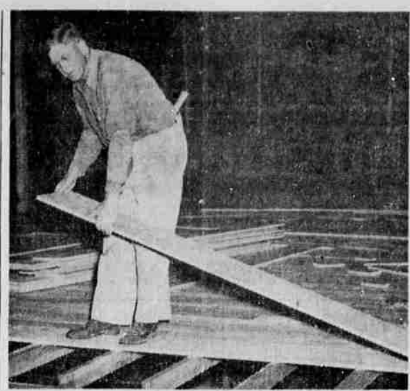
MAY FETE TO BE ENACTED FROM SPECIAL STAGE —Jim Mess, above, maintenance man for School District 4, supervised and did most of the construction on the specially built stage set up in front of the grandstand at Finlay Field. Nearly 600 students from Senior High and Roseburg grade schools will participate in tonight's show—reportedly the first of its kind here.
