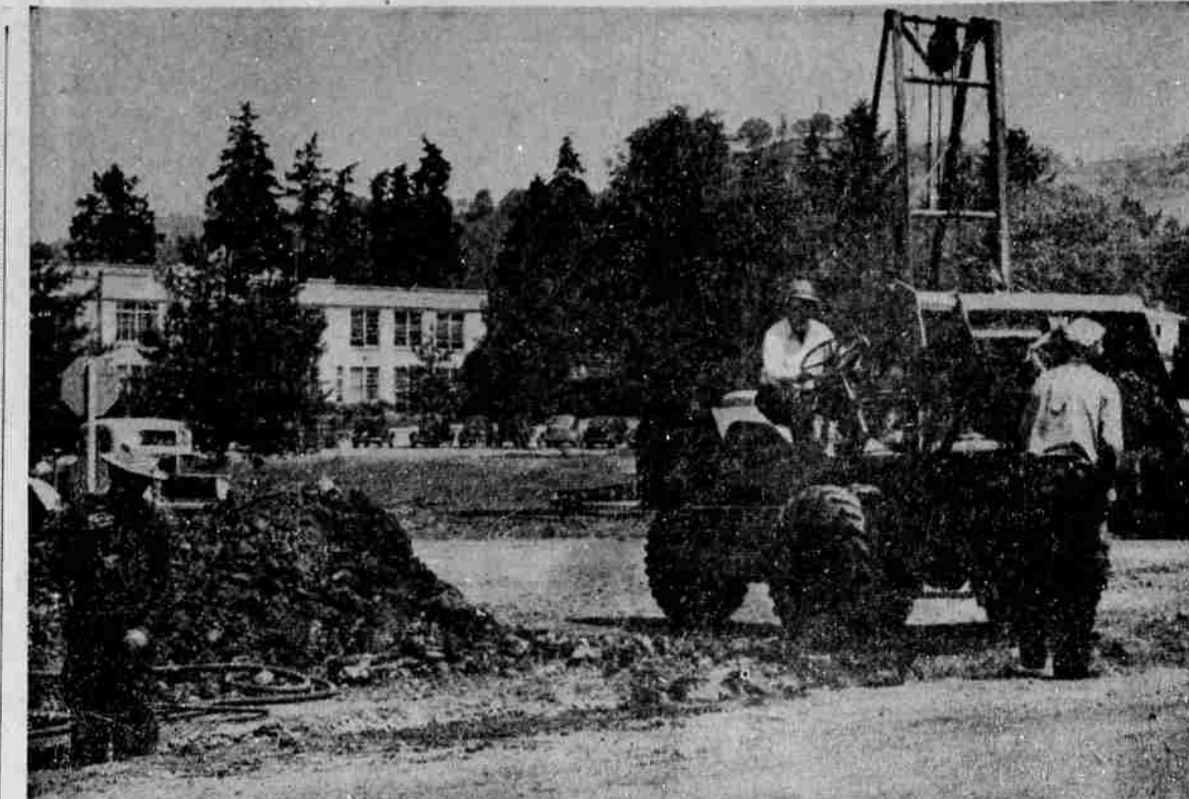
CABLES UNDERGROUND—Telephone company workmen this week laid their wires underground in four-division conduit across school property along Harvard Ave. Removal of the overhead lines was necessary because of the Fullerton School building expansion, which interfered with the lines.
