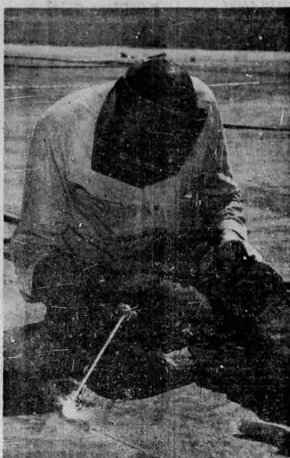
GUESS WHO—No, it isn't the phantom. The masked man in this picture is Jack Hayes, California Oregon Power Co. welder, working on the company's new reservoir on the hill north of town.
