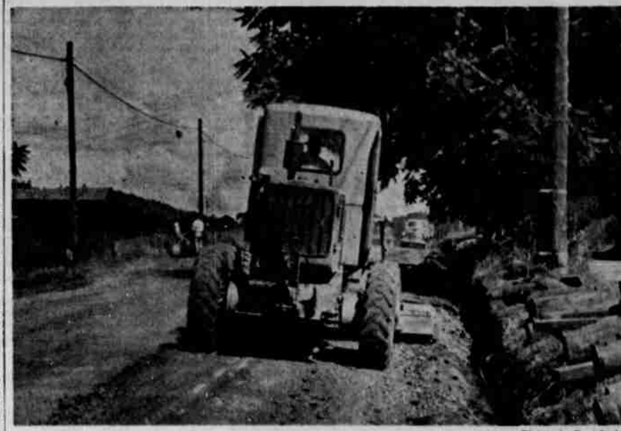
HARVARD AVENUE WIDENING—County road crews this week began construction work on the widening of the two block section of Harvard Avenue from the west city limits to Harrison Street. The street is being widened to a 35-foot width. The side lanes will be paved, and concrete curbing are to be installed. Some of the curbing work has already been started. Drains will also be laid.
