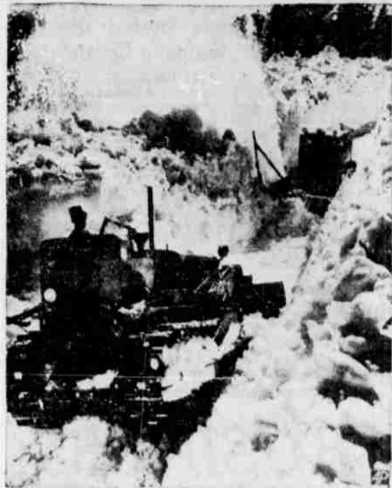
SNOW CLEARED FROM ROAD —Snow removal on Lassen Peak Highway near Mineral, Calif., is progressing past the spot where the annual midsummer ski tournament sponsored by the Mt. Lassen Ski Club is held. With an extra powerful bulldozer pushing the top layer of snow to one-side, a rotary snow plow blows it away. Drifts as high as 30 feet have delayed opening of the road. (AP Wirephoto)
