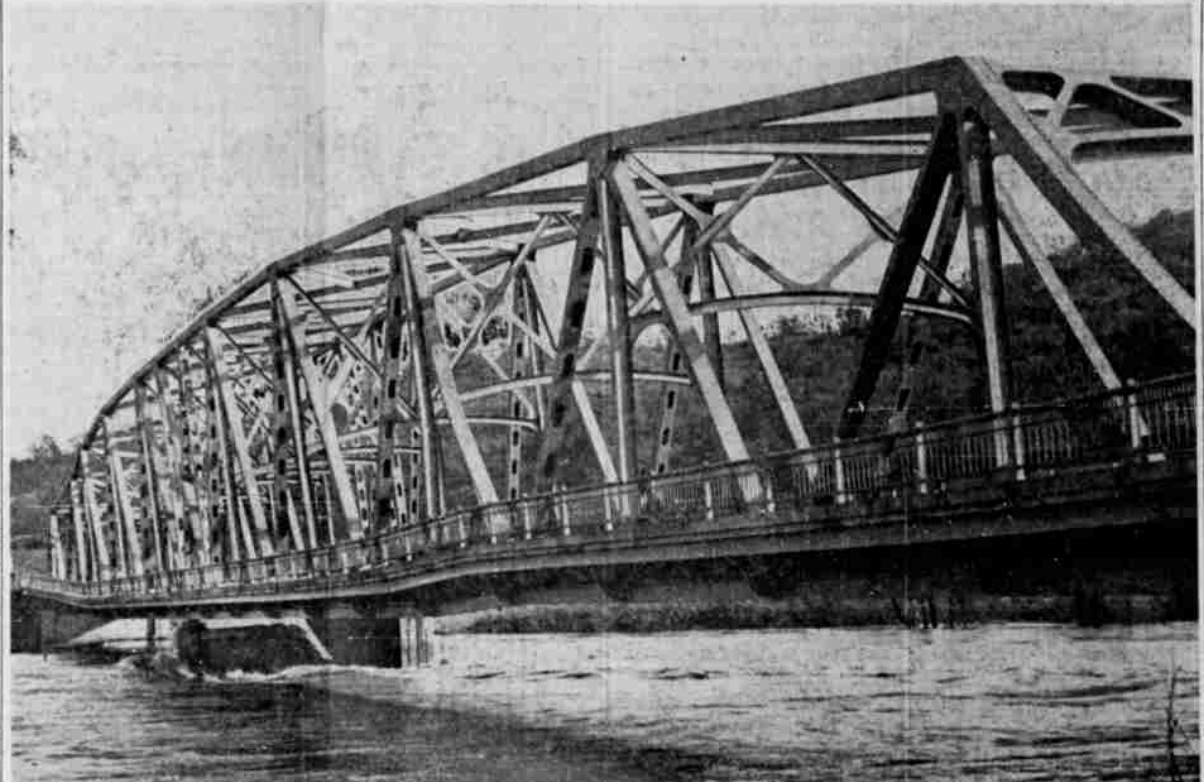
HIGHWAY BRIDGE DAMAGED —This is the Pacific Highway bridge four miles south of Dillard, which received a severe battering from the South Umpqua River during Tuesday night's storm. The upper view is taken from the up-river side, showing the twisted girders of the super-structure. View at right shows the center pier, split in two by the river's swift currents. Additional flood pictures may be found on Page 2.
