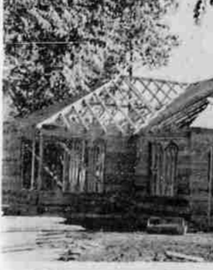
LOCATION JUST TO HIS LIKING—This is the six-room home Cliff Aten is building for himself on Lilburn street in Laurelwood.
