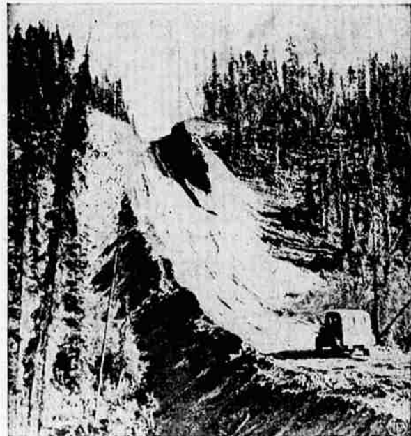
Workers on the new "Alcan" military road across Canada to connect the U. S. with Alaska are making rapid progress as they equalize topography by cutting through hilltops, such as that shown above. The road, which will be a major factor in the defense of Alaska, will be sufficiently completed for all-way travel by trucks by December 1, authoritative sources declared.
