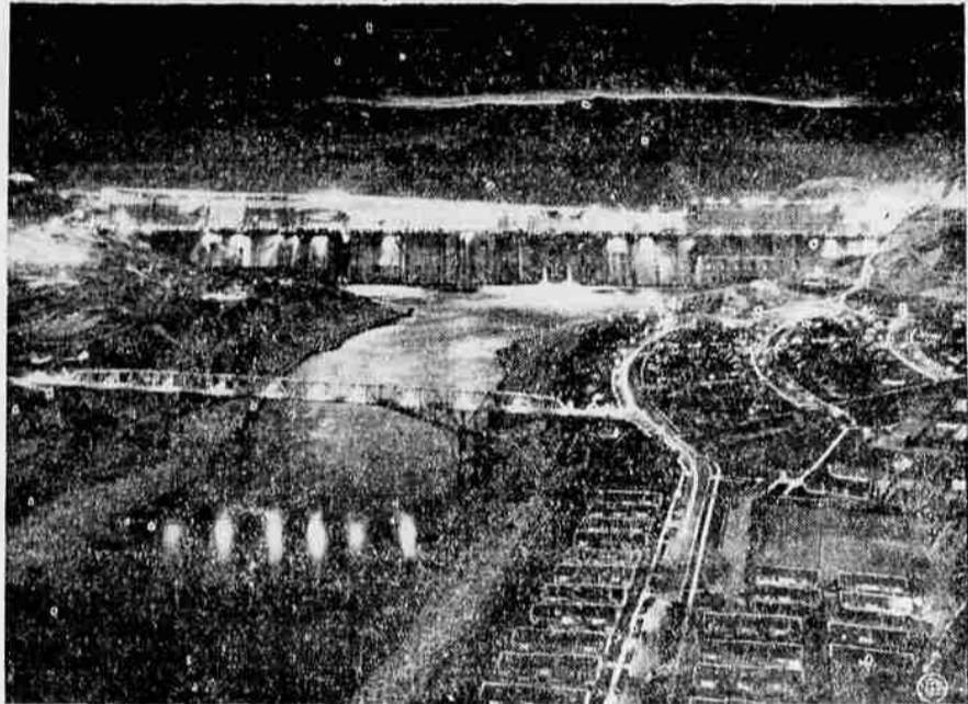
Night falls, but work continues under a battery of lights at Grand Coulee Dam in Washington, where the mighty structure is rapidly being rushed to completion. By the end of this year the first power will be available from two 10,000-kilowatt power units.
