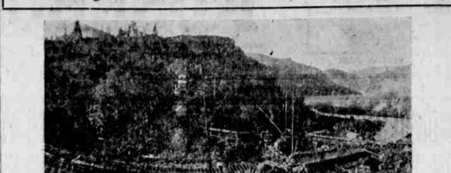
Copco No. 2. Upper photo shows dam site, quarry, concrete mixing plant, by-pass flume and tramway for handling concrete. Intake of portal of Tunnel No. 1 can be seen through tramway. This view was taken January, 1925.
